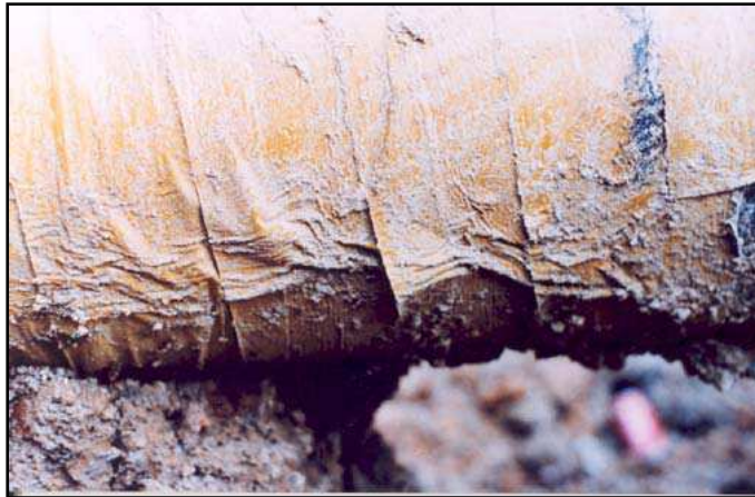
SOIL STRESS FAILURE
